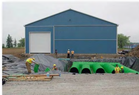
Subsurface HDPE arched chamber system
