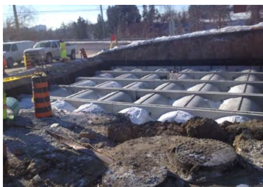
Subsurface concrete arched chamber system
