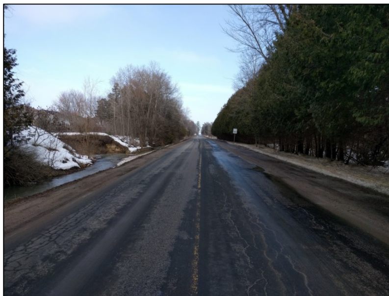
Figure 6: Existing 7 th Line Pavement Structure Deterioration
