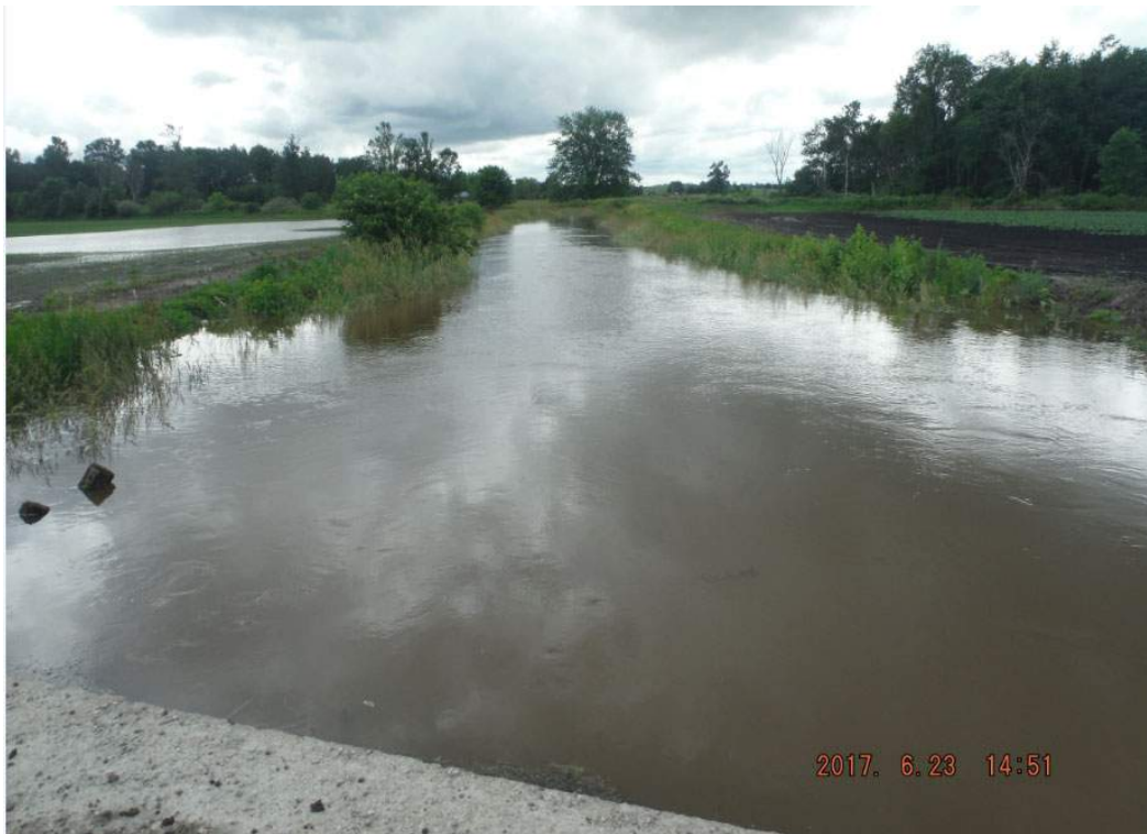
Figure 8 Existing Drain June 2017 Flood Event – Main Drain at STA. 4+359
