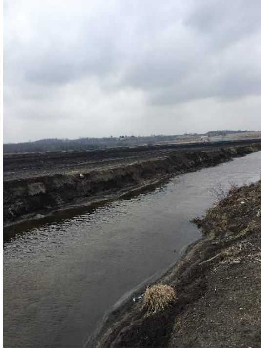
Photo 21: Looking east, the Drain with eroded, non-vegetated banks.
