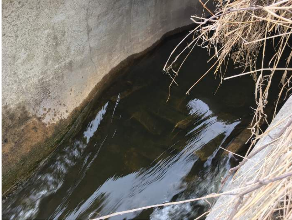
Photo 7: Looking east, the wooden planks within the outlet of the single CSP beneath Highway 400 (April, 2018).
