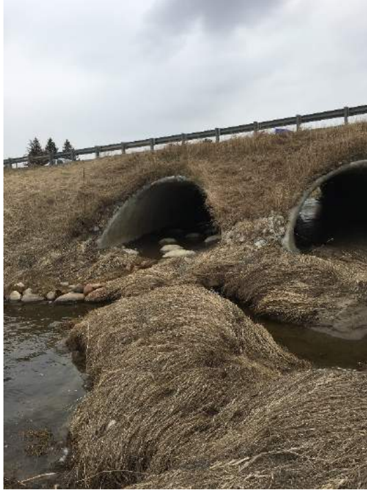
Photo 9: Looking east the outlet of the double shot-creted CSPA culverts beneath Highway 400 (April, 2018).
