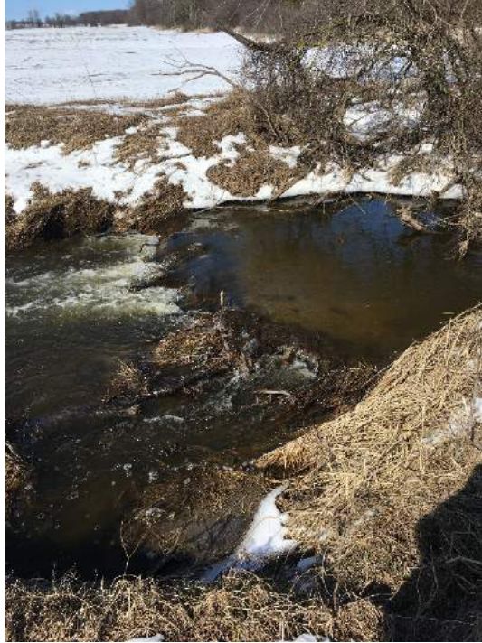
Photo 31: Looking west, debris dam present upstream of the eroded bank and upstream of 4 th Line (April, 2018).
