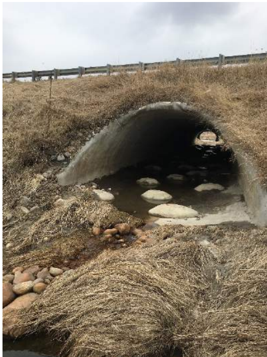
Photo 10: Looking east, the concrete lined CSPA with artificial boulders constructed through it (April, 2018).
