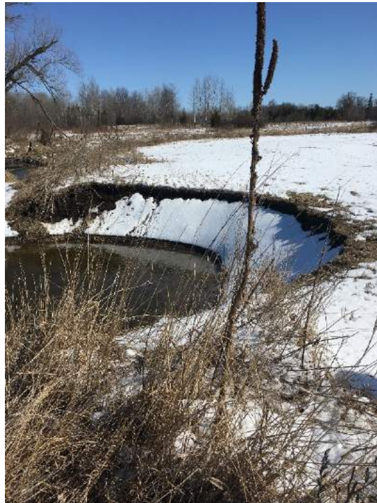
Photo 30: Looking north, highly eroded bank present on the right upstream bank of the Drain upstream of 4 th Line within agriculturally cultivated land (April, 2018).
