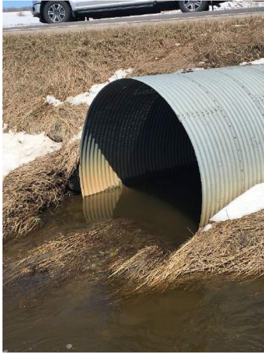
Photo 27: Looking north, the outlet of the overflow CSP culvert located beneath 4 th Line (April, 2018).
