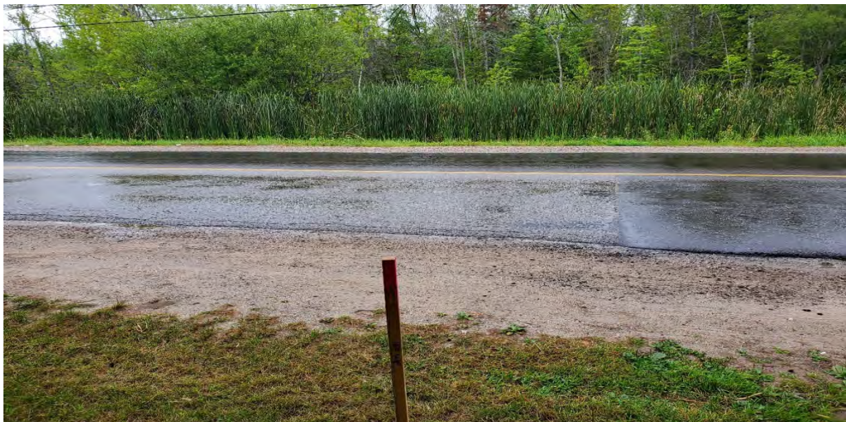
Figure A.6: 25 th Side Road, off shoulder, facing west. Showing low to medium severity edge cracking, slight wheel path rutting, medium severity patching, low to medium severity construction joint cracking. [CS, August 2021]
