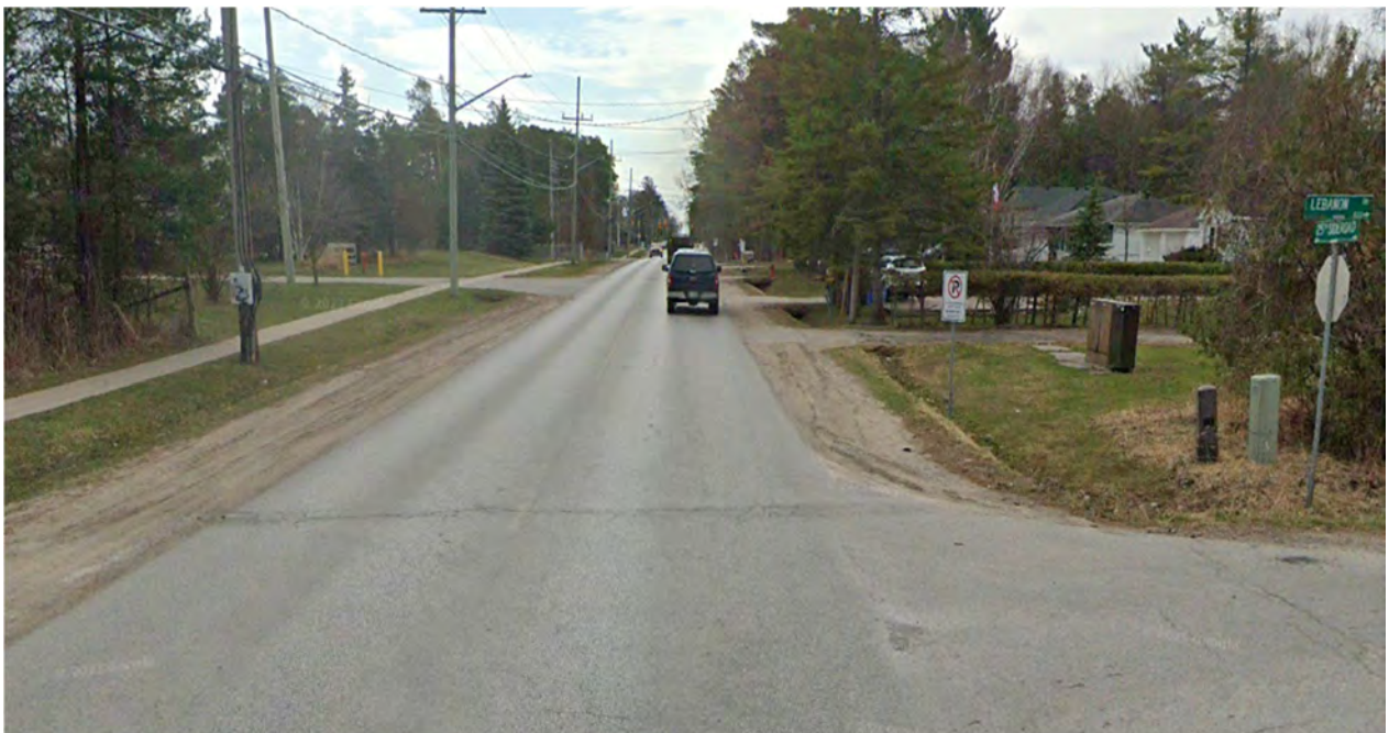
Figure A.4: 25 th Side Road, northbound, facing north. Showing low to medium severity longitudinal/transverse cracking. Low severity raveling and coarse aggregate loss. [CS, August 2021]
