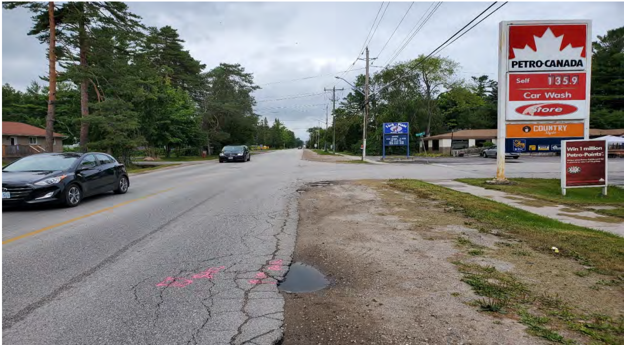
Figure A.5: 25 th Side Road, northbound, facing north. Showing medium to high severity edge cracking associated with medium severity alligator cracking. [CS, August 2021]
