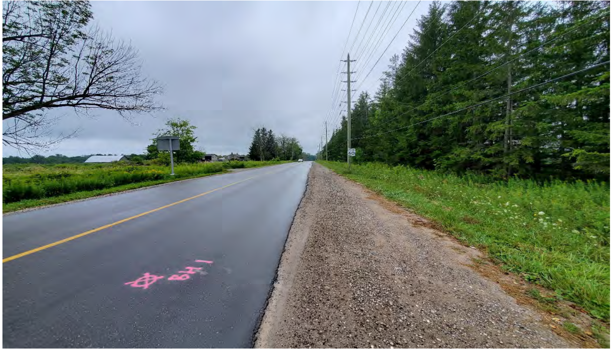
Figure A.7: 25 th Side Road, northbound, facing north. Showing low severity edge cracking. [CS, August 2021]
