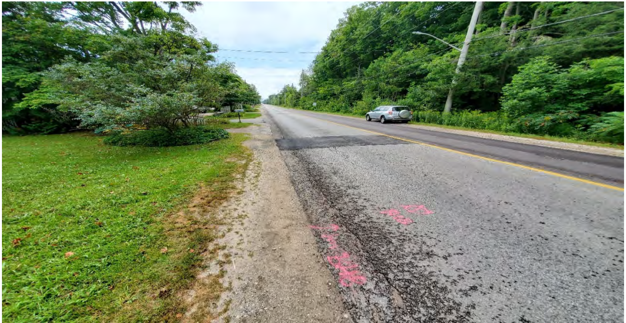
Figure A.3: 25 th Side Road, southbound, facing north. Showing frequent medium to high severity edge cracking associated with medium to high severity raveling and coarse aggregate loss. Medium wheel-path flushing. [CS, August 2021]
