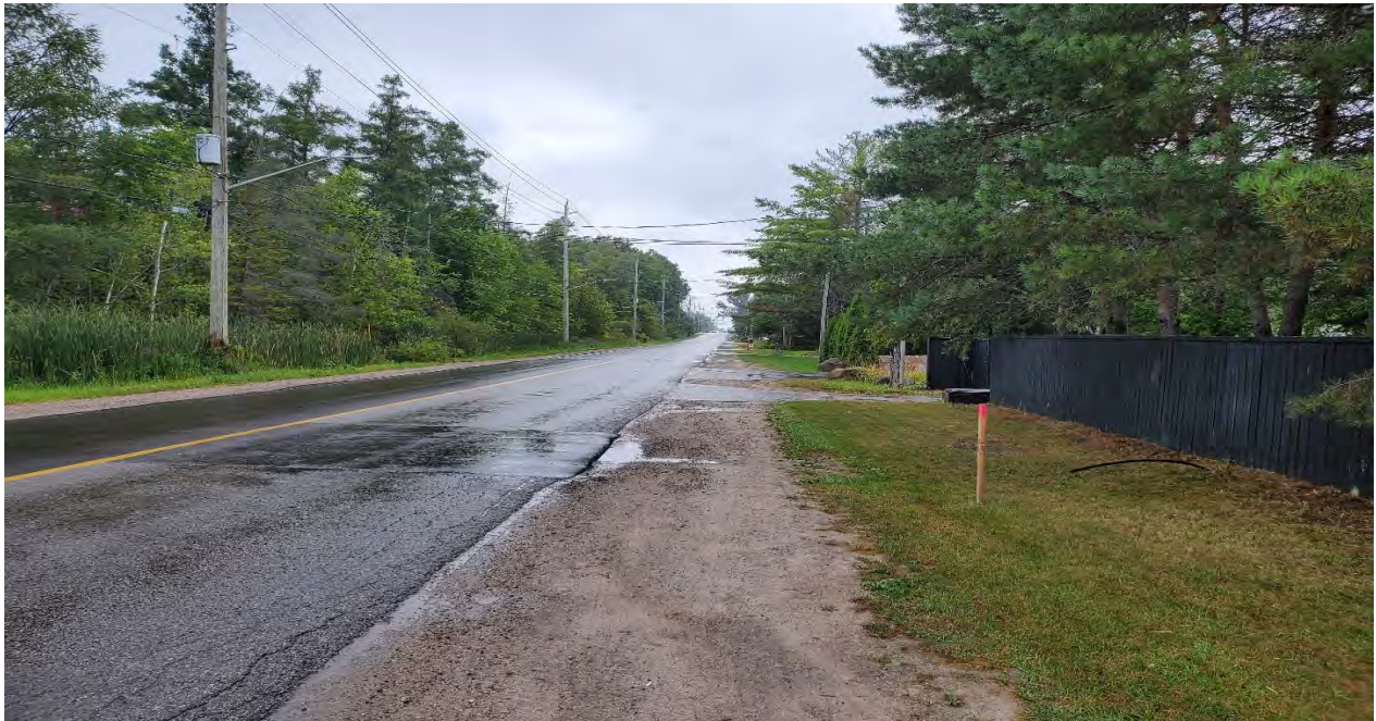
Figure A.1 25 th Side Road, northbound lane, facing north. Showing frequent medium to high severity edge cracking associated with medium severity transverse construction joint cracking along asphalt patch, slight wheel-path flushing. [CS, August 2021]
