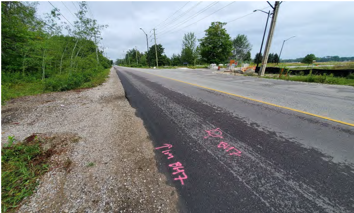
Figure A.9: 25 th Side Road, northbound, facing south. Showing frequent low to medium pavement edge cracking associated with medium to high severity ravelling and coarse aggregate loss. Medium wheel-path flushing, slight wheel path rutting. [CS, August 2021]
