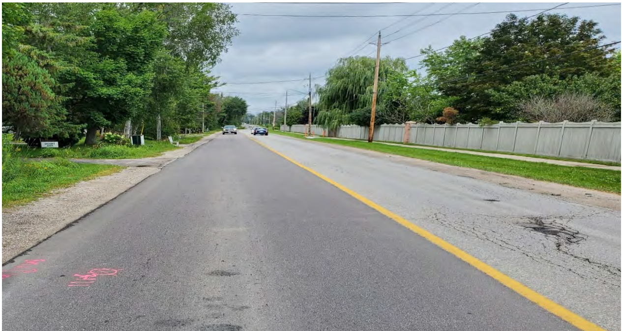
Figure A.2 25 th Side Road, southbound, facing north. Showing medium to high severity alligator cracking and potholing, frequent slight wheel-path flushing, medium severity ravelling and coarse aggregate loss. [CS, August 2021]
