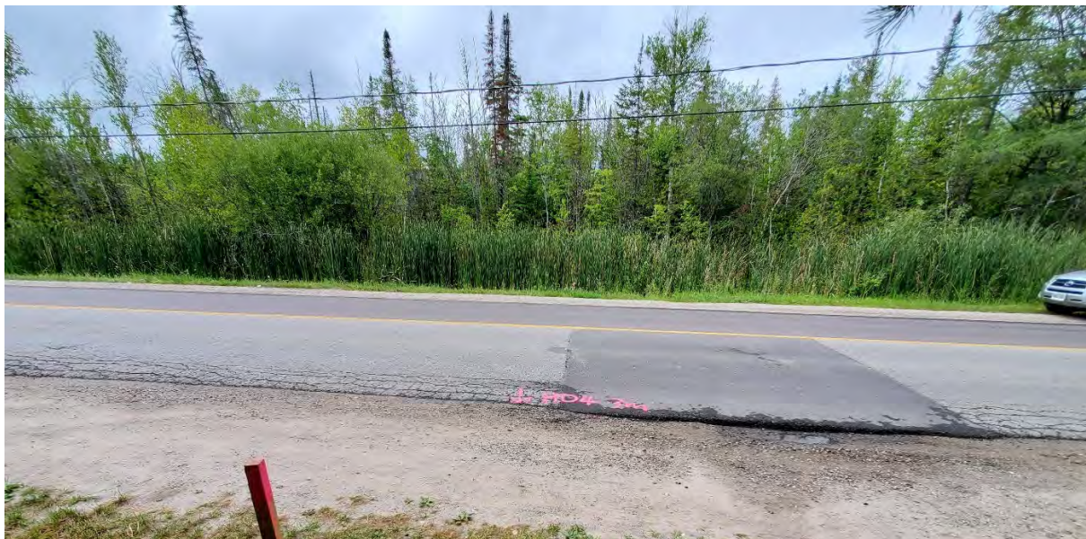
Figure A.10: 25 th Side Road, east off-shoulder, facing west. Showing frequent medium to high edge cracking associated with medium severity transverse construction joint cracking along asphalt patch. Medium severity patching and medium to high severity alligator cracking. [CS, August 2021]
