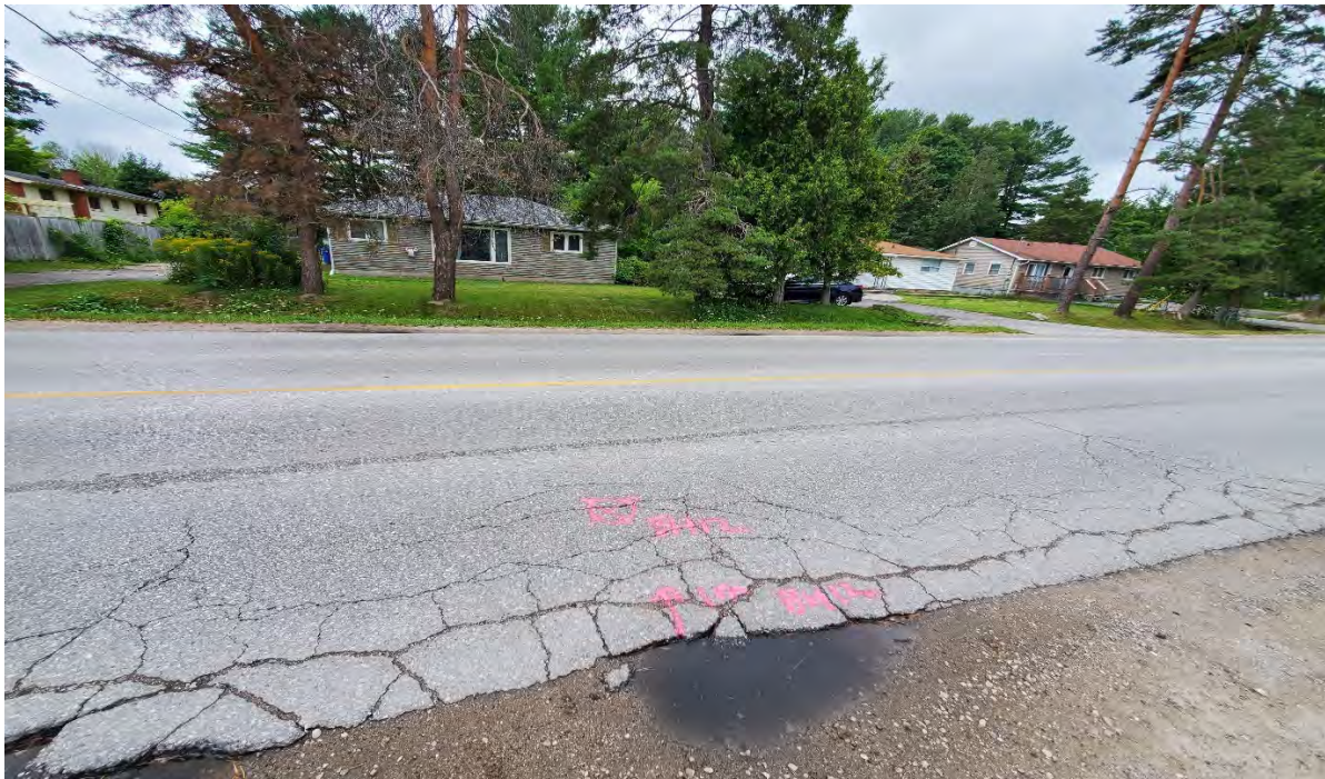
Figure A.11: 25 th Side Road, southbound, facing east. Showing medium to high severity edge cracking, medium severity alligator cracking, medium severity ravelling and coarse aggregate loss. [CS, August 2021]
