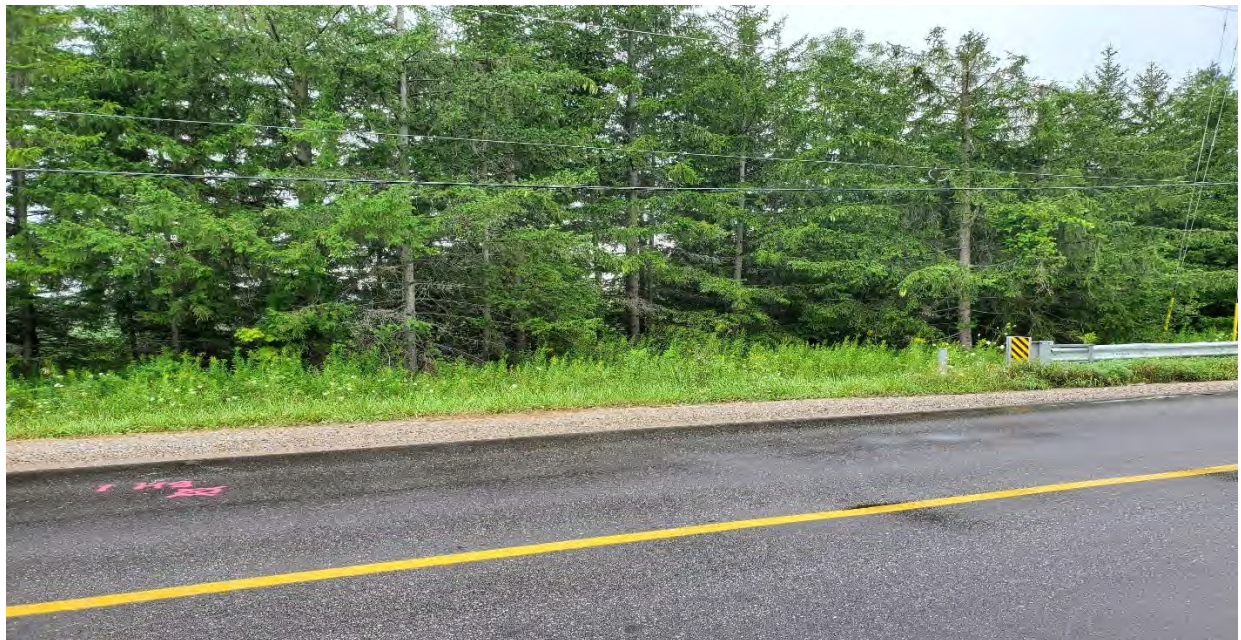
Figure A.8: 25 th Side Road, northbound, facing west. Showing medium severity ravelling and coarse aggregate loss, slight wheel-path rutting and low severity longitudinal and transverse cracking. [CS, August 2021]
