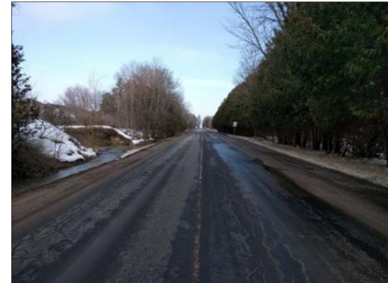
Existing Pavement Structure Deterioration
